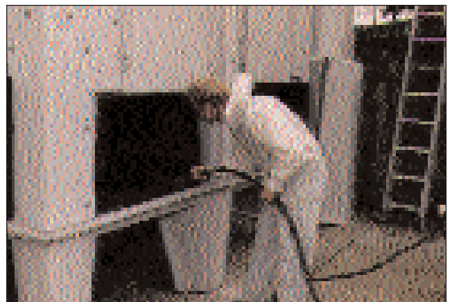
▲ No need to enter confined spaces to clean basins.
